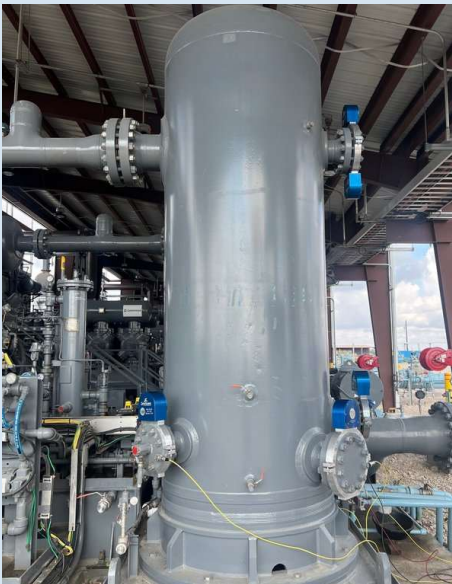
Rohr Dampers Installed on Suction Scrubber
